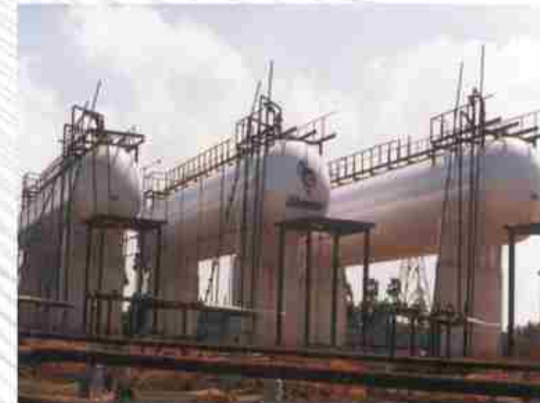
Bullets – Mounded Storage & Above Ground Bullets
